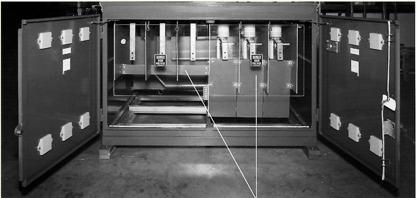
Low-Profile Switchgear Cabinet
