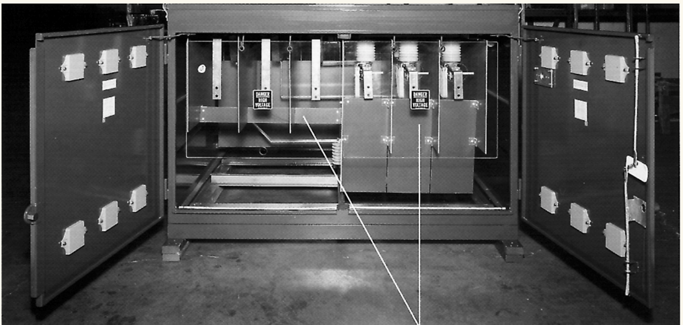
Low-Profile Switchgear Cabinet
